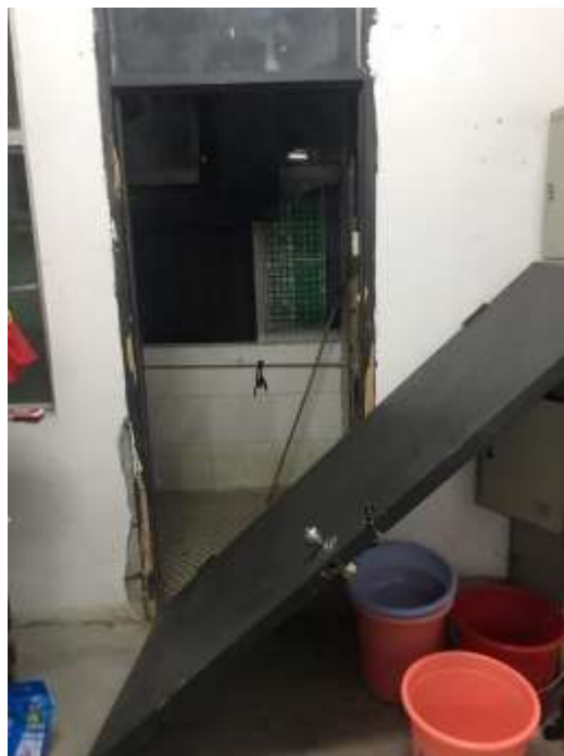
(the blown down door)
