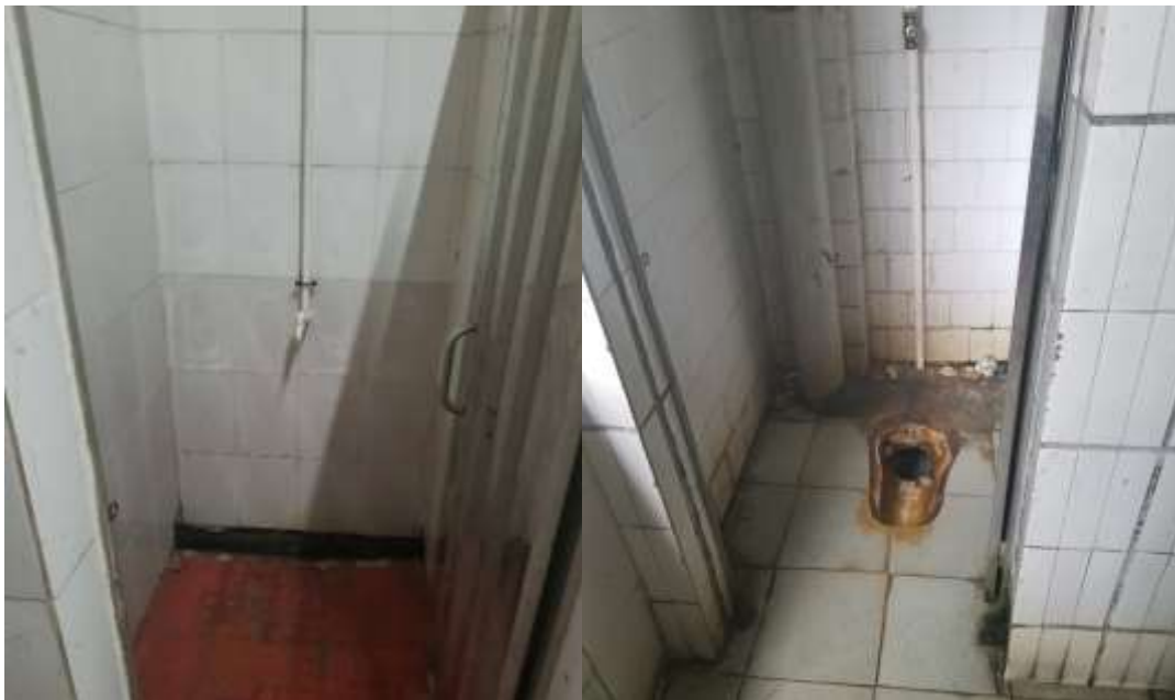
(The bathroom and shower room are small and dirty)
