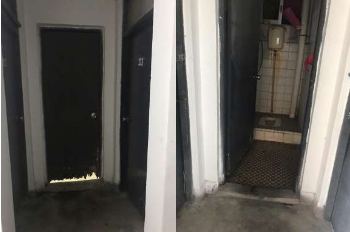
(Left: the bathroom doors are broken; Right: there is only one squat toilet in the bathroom)
