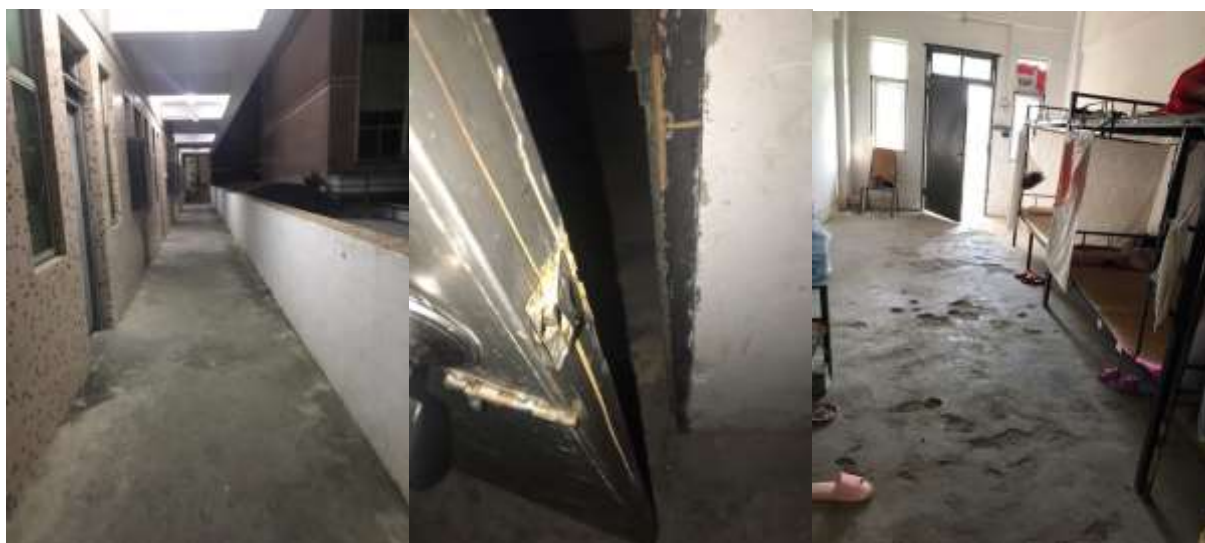
(Left: the dormitory corridor; Middle: the door of the dormitory room; Right: the room is messy and the floor is broken)
