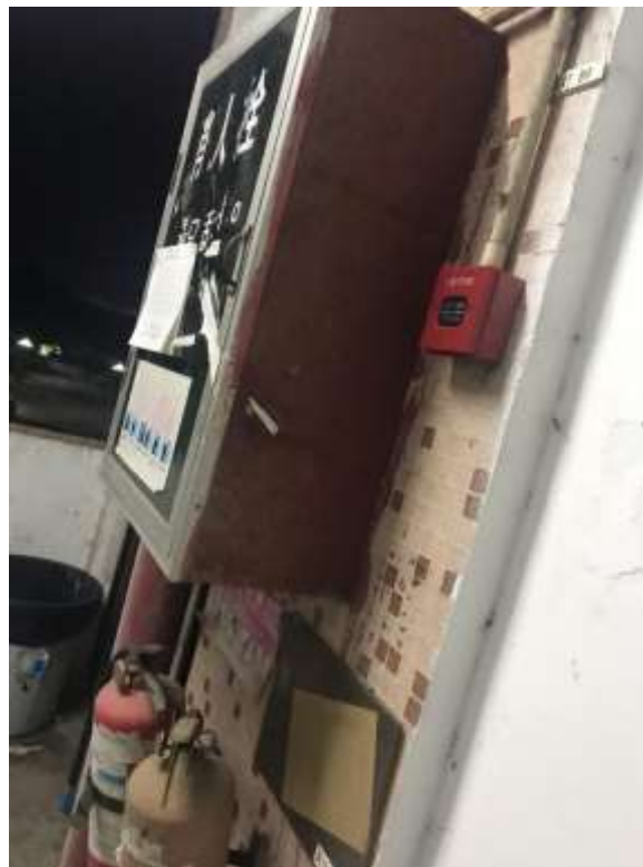
(A fire extinguisher in the corridor)
